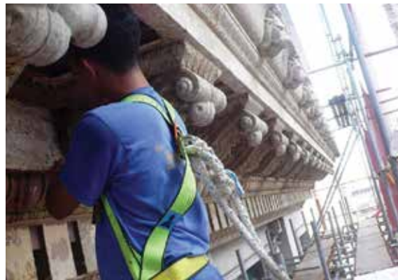
Worker meticulously cleaning, repairing, and restoring the building’s exterior moldings and ornaments.
