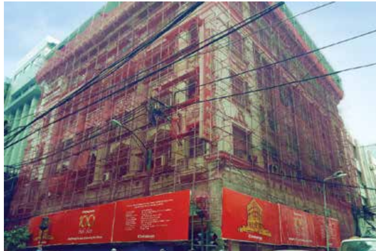
Steel scaffoldings surround the building for the painstaking work of restoring the ornate moldings, iron grills, and other exterior architectural details.
